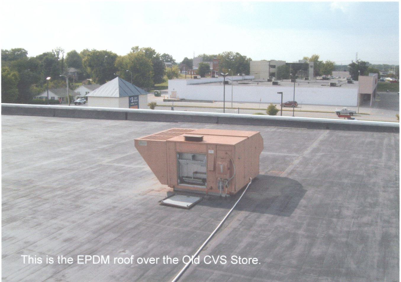
It looks like the insulation was installed over a damp roof surface.
